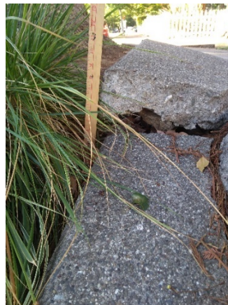
Fig. 2. 2019/2020 Grand Jury. Close-up of the same displaced sidewalk, showing a displacement of eight inches. 2020.
